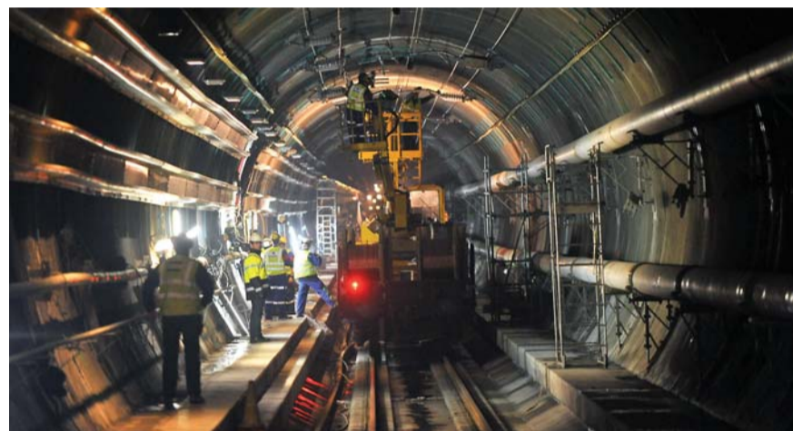
Top: Channel Tunnel fire damage, 2008. Bottom: Kent FRS and French firefighters confer during Channel Tunnel fire, 2008.
